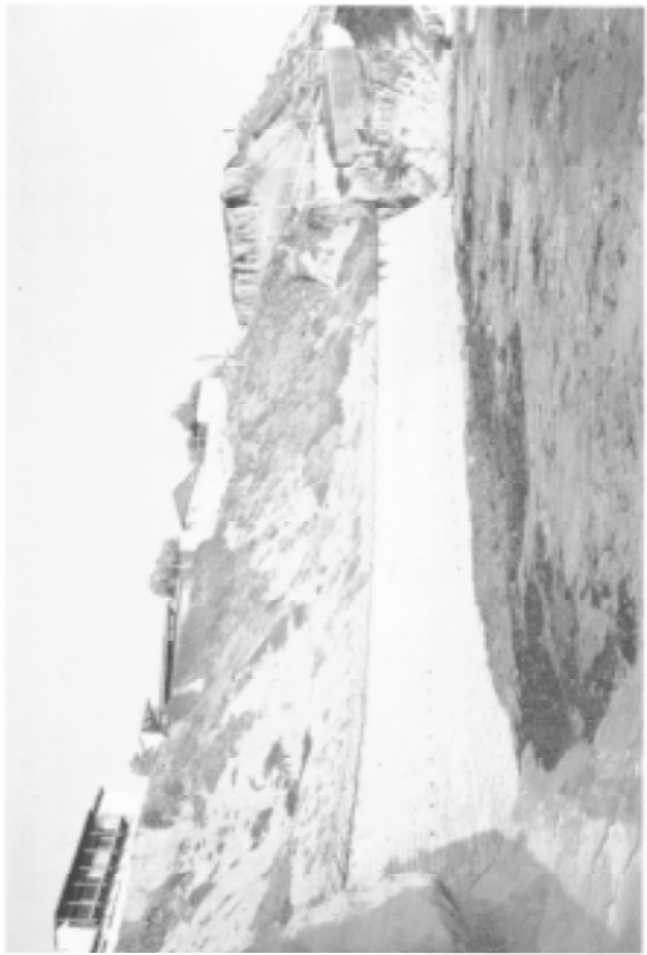
Figure 3.7. Helping erosion: running storm sewers on the cliff (Del Mar). Slowing erosion: building a sea wall (Solana Beach).
